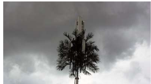
FIG. 1: This cellular tower/palm tree combo monstrosity is exactly the type of eyesore Cellular Charm is looking to eliminate with its tower models.
