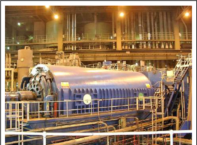
FIG. 5: Manufacturing facilities for power-plant turbines are enormous and involve highly technical work in their construction.
